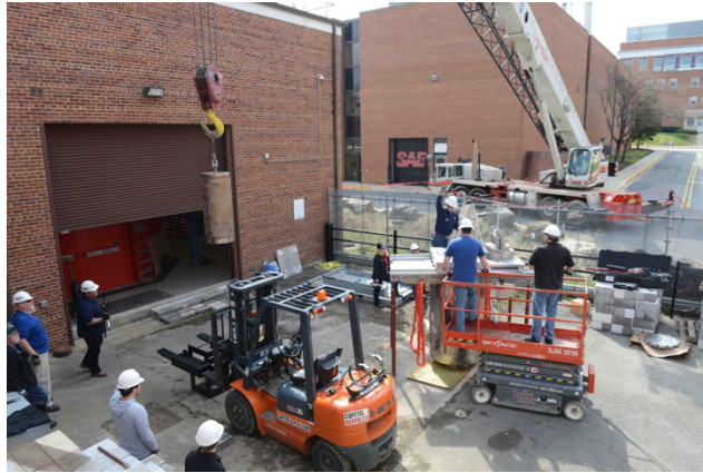
Figure 3: Fuel is transferred from a shipping cask to the MUTR in March 2017.
