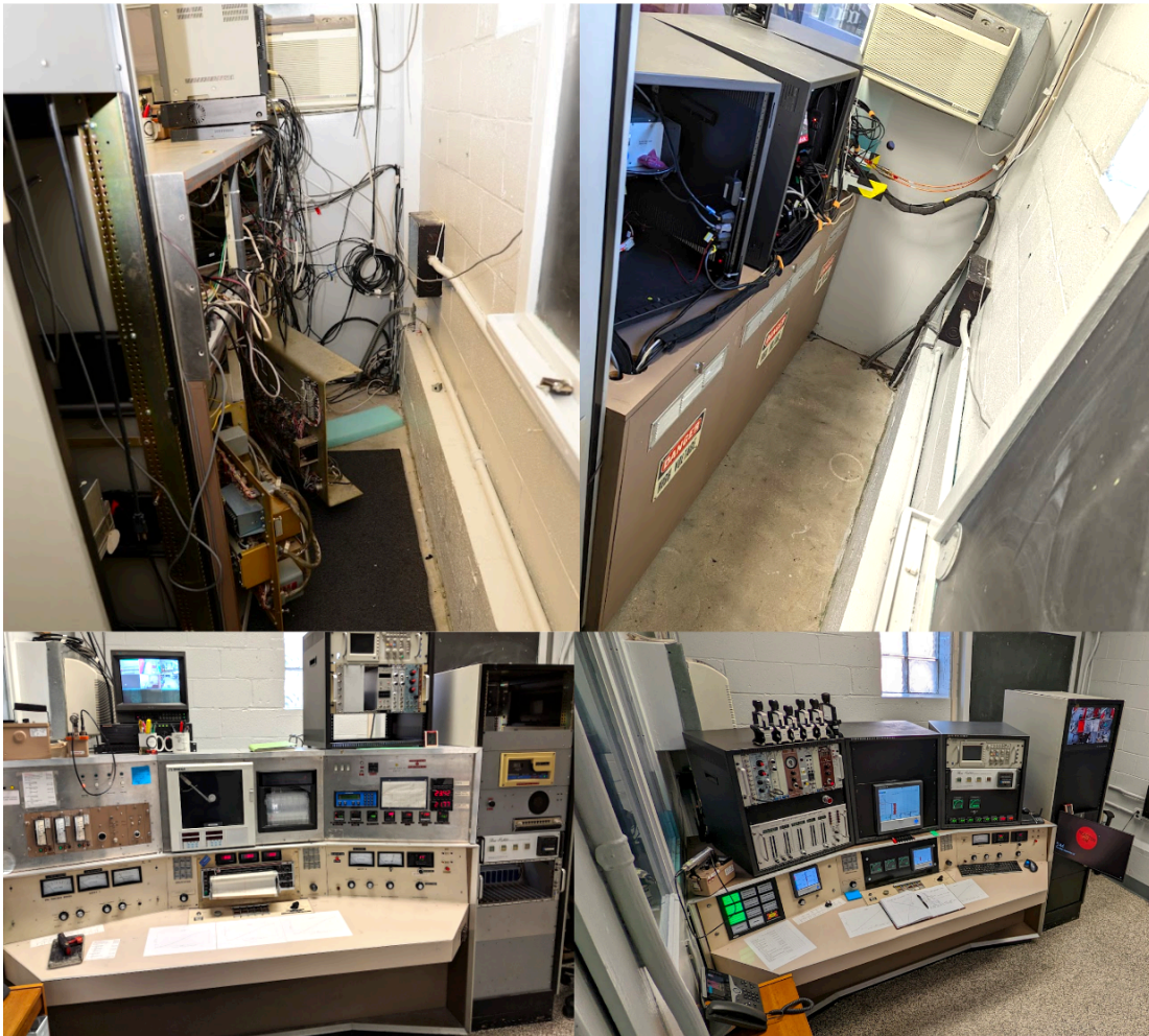
Figure 5: The MUTR Console before (left) and after (right) upgrades.
