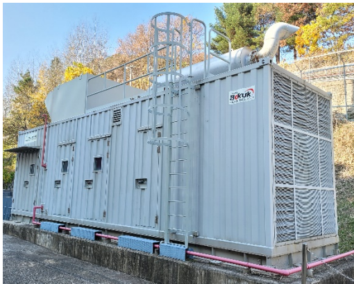
Additional emergency diesel generator
