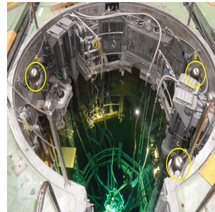
Pool Radiation Monitoring System
