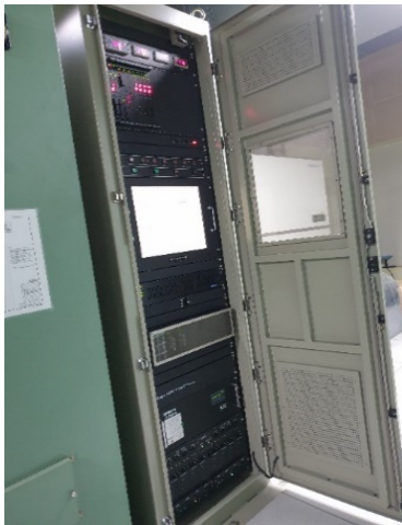
Seismic Monitoring System
