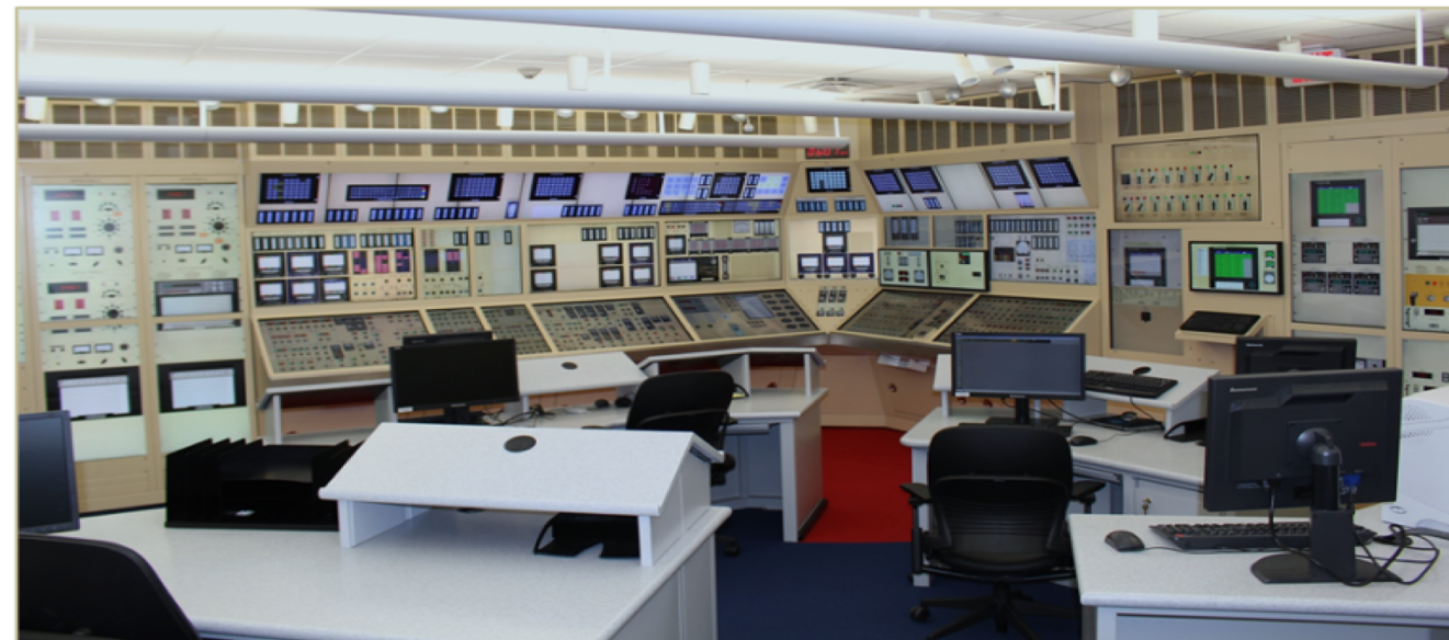
Touch Screens Control Room Panel
