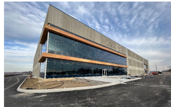
Photo of new >60,000 sq ft facility under construction for global investigational & commercial therapeutic RP supply (expected 2025-2026)
