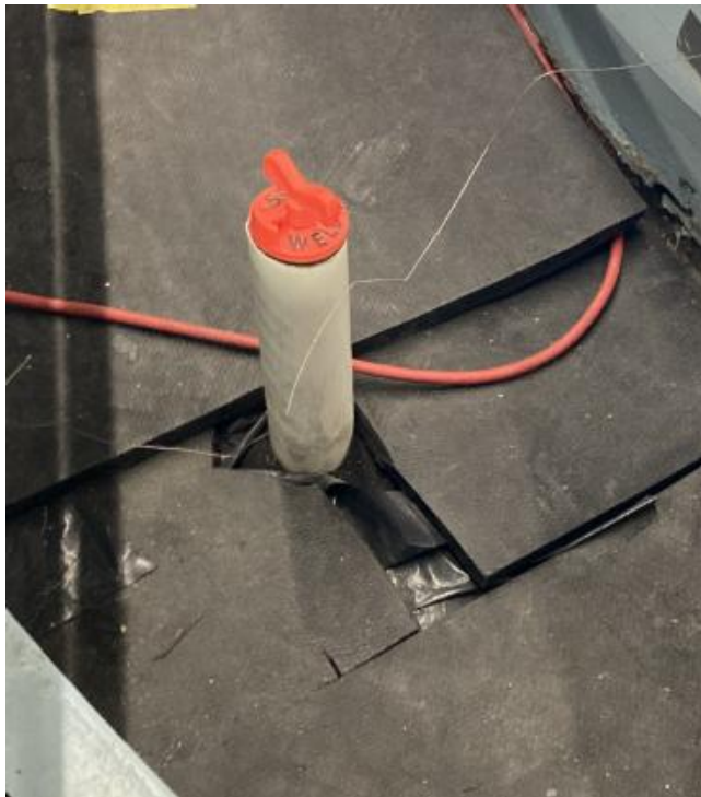
Monitoring well of the space between tanks
