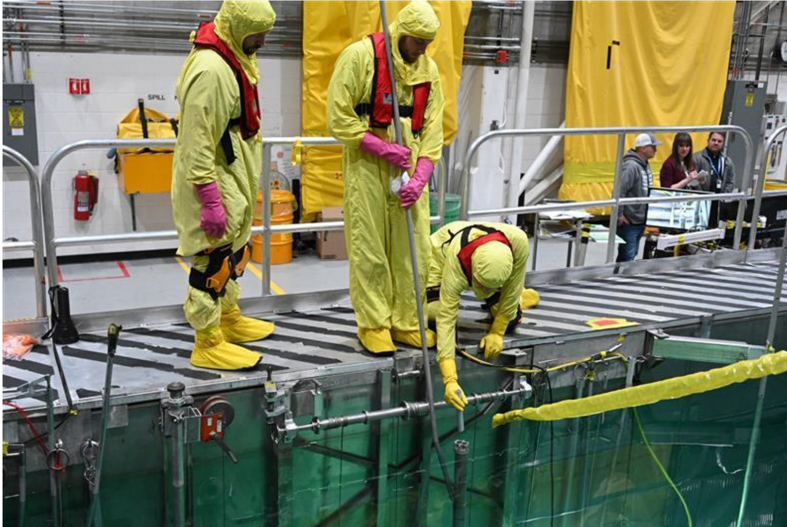
ATR operators working with the MP-2 South Flux Trap experiment.
