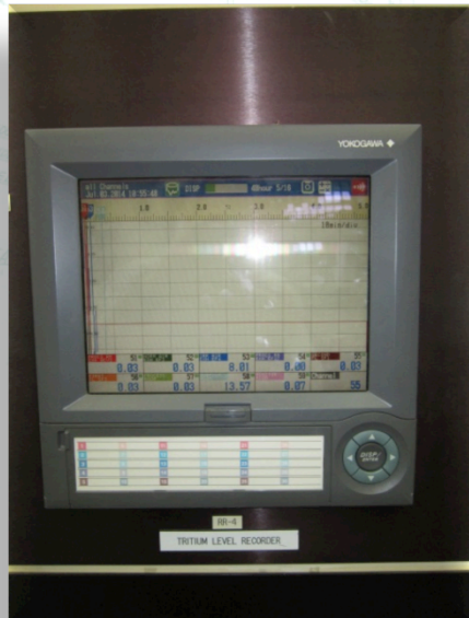
Control Room Recorder
