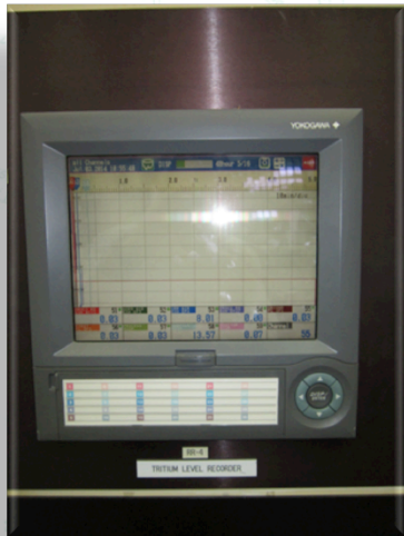
Control Room Recorder
