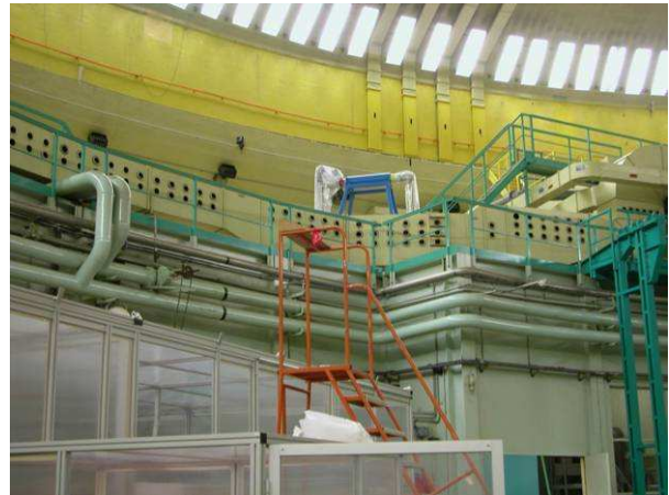
Figure 4 – View of part of the networks to be diverted prior to phase 1 of the dismantling operations
