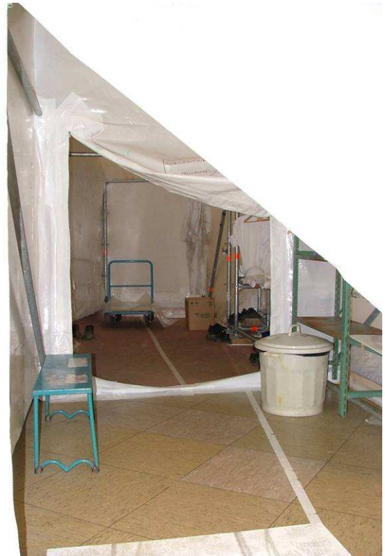
Figure 10 – View of personnel access air lock
